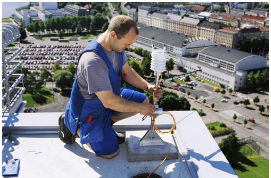
A WXT520 being installed at the top of the 72-meter tower at the Olympic Stadium in Helsinki, Finland.
